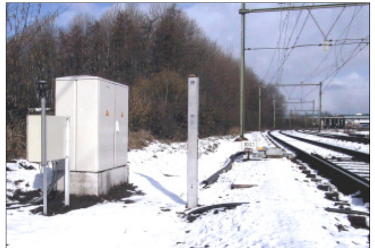
METEOSCAN installed near Utrecht (The Netherlands).
