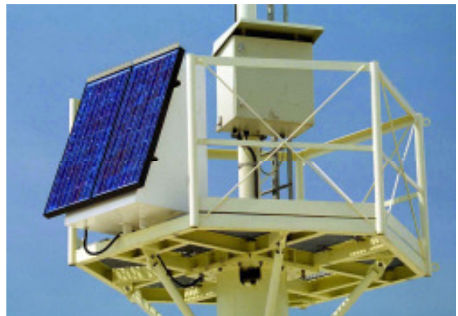
SOLAR CUBICLE SK-10 mounted on Dutch weather station
