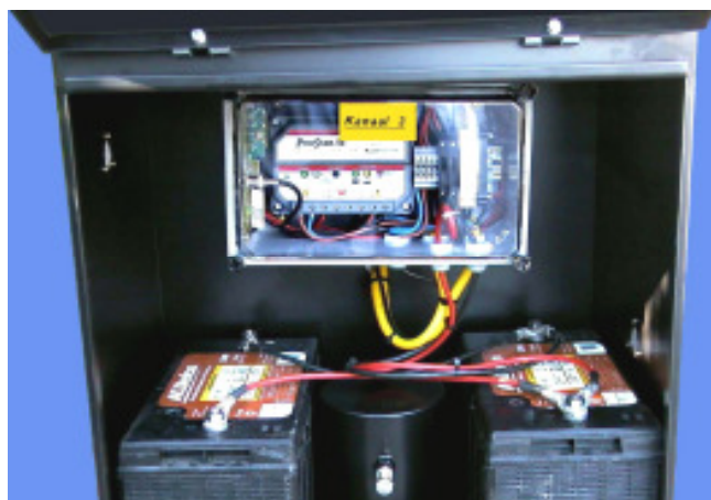
PROSTAR 15 installed in solar energy unit
